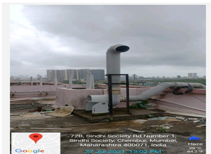
Fig. Exhaust of Fume hood installed in VESIT Chemistry Lab
